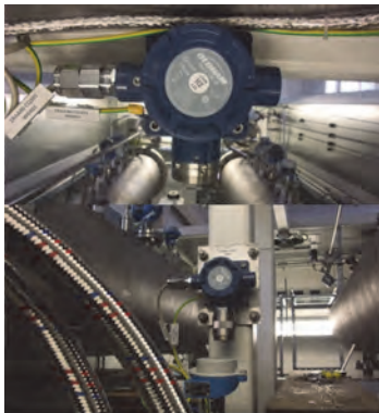
H 2 - & O 2 -transmitter integrated and operable in the AEL-demonstrator facility
