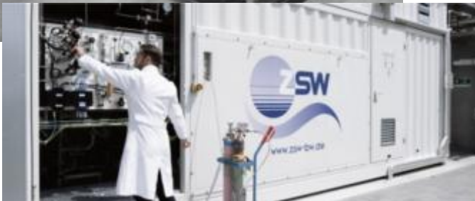
Electrolysis system (1 MW el )
