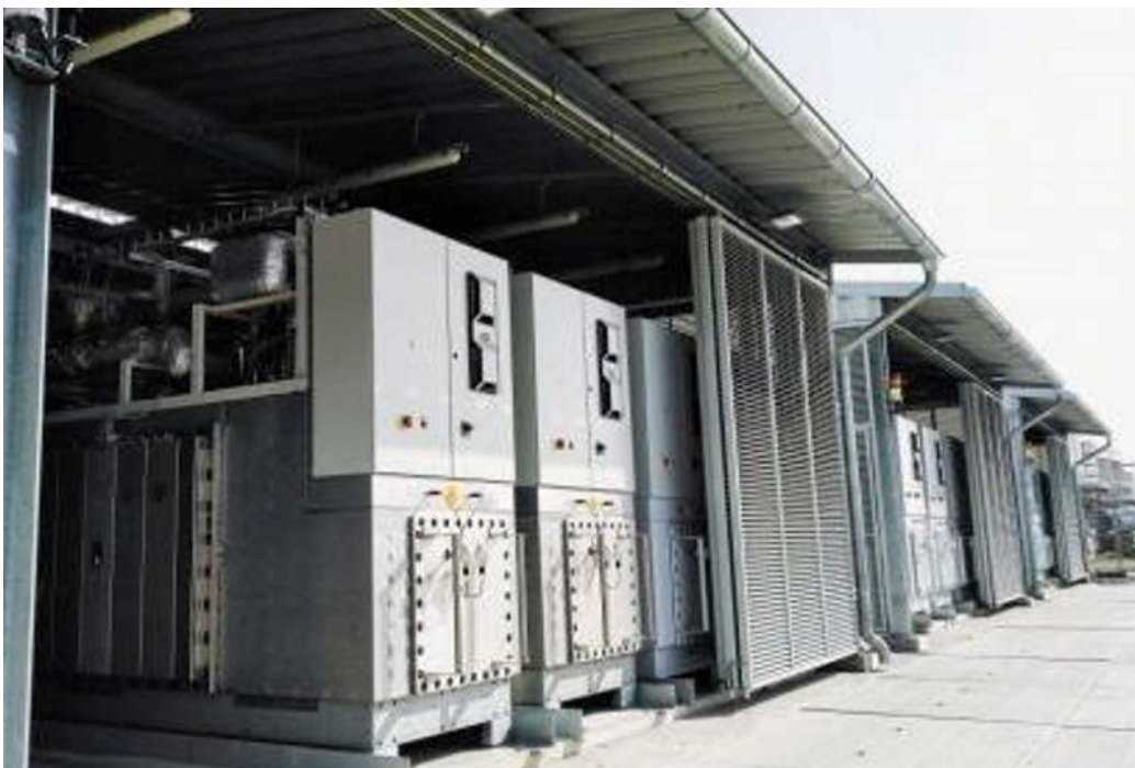
2,6 MW Sunfire @ Neste Biofuels Refinery Rotterdam, NL
